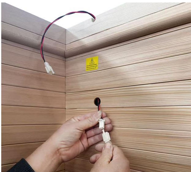
(9) Connect sauna light cable as above.
